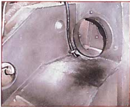
Fig. 7 - Bilge Fan Installation Location (Engine Compartment)
