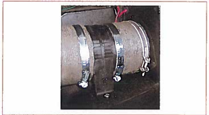
Fig. 8 - Bilge Fan Unit Installed (Engine Compartment)
