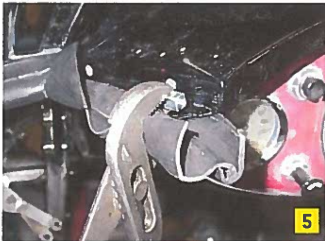
Photo 5: Use a channel-lock pliers, with one jaw under the rivet head, to squeeze the block down, thereby flattening the rivet tips against the metal flange.
