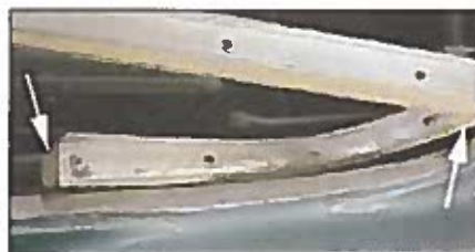
Photo 23 - The white vinyl should completely cover the wood blocks with tight gaps where the edges meet (see arrows). Lips on the aluminum facing strips are for mounting the rubber seal strips.
