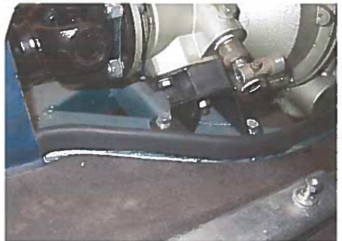
Photo 21: The second step is to use contact cement again to adhere the strip to the outer face of the metal flange. Make sure the rubber layer is tight to the metal to keep the overall thickness at the folded edge as thin as possible.
