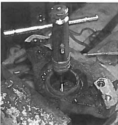
Tapping a hole in the piston in order to fit a grease nipple
