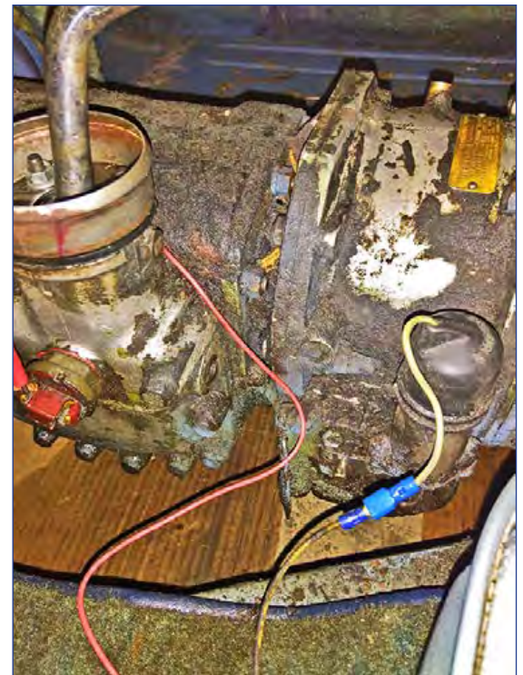
Jumper wire going from the gear box switch "input" to the OD Solenoid (going around the shift lever to keep it away from the spinning drive shaft. This essentially bypasses the gear box OD switch.
